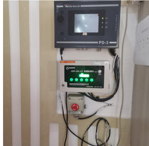
储罐泄漏检测仪
