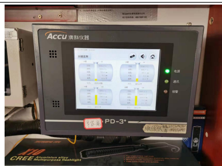
储罐监测液位仪
